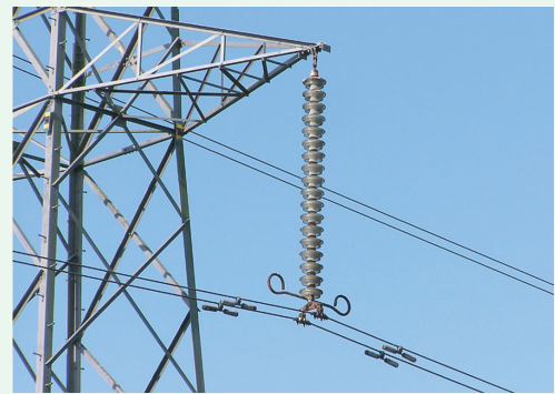
Figure TF26-5: Cap and pin insulator string (the vertical string of discs) on a 275 kV suspension pylon.
